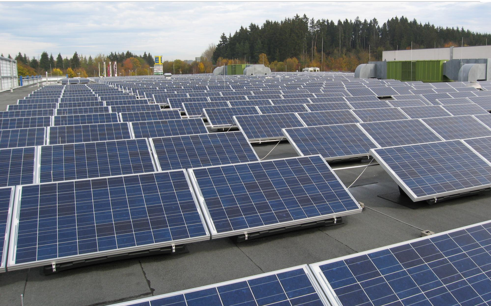
Edeka Supermarket, Bad Dürrhein, Germany by Sunways AG - 290 kWp
